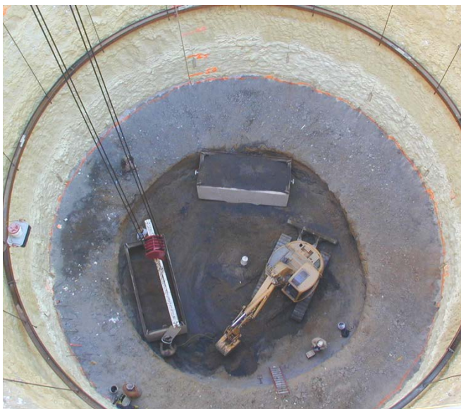
JCK Underground staff provided program, construction and design management for the NBC CSO Program (above and below).
