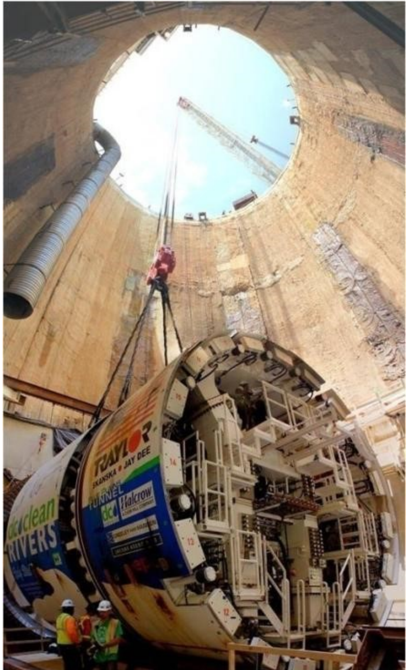
JCK Underground staff provide program management services for DC Clean Rivers Project.
